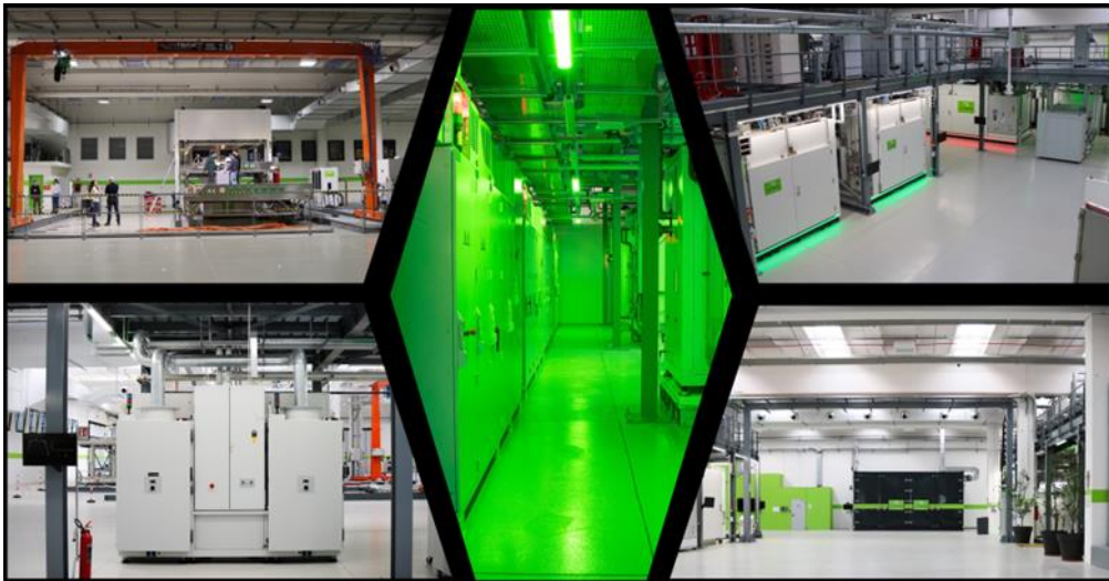
Figure 11: Pictures from REINOVA's facility
